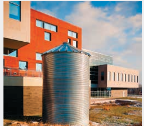
Stormwater collection cistern at East HCT
